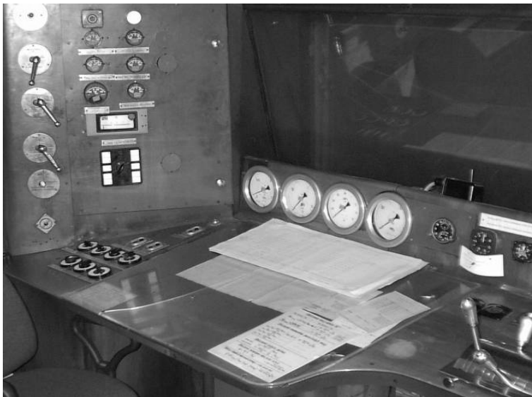
Fig. 5.3. Control room – inside. Control devices and gauges
