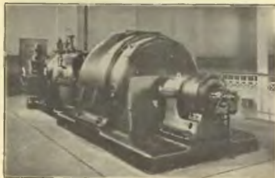
Turbogenerator 2.200 KW z odbiorem pary.
