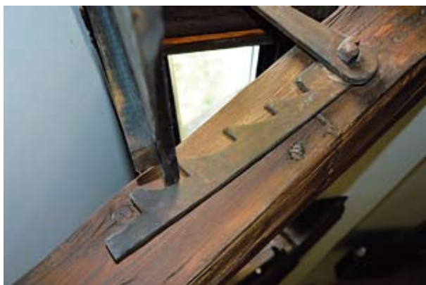
Fig. 53. Flaps for regulating air flow. Photo by A. Fortuna-Marek
