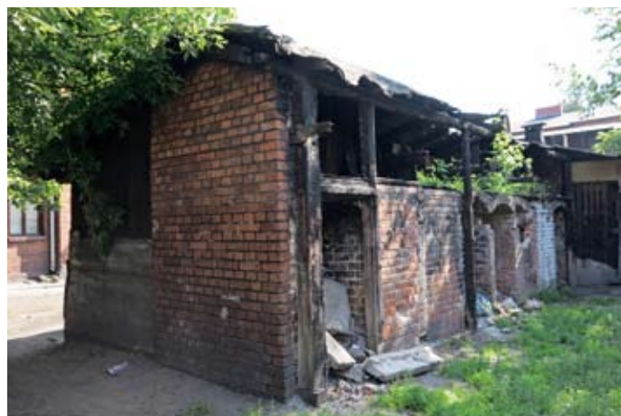
Fig. 59. An endangered outbuilding. Photo by A. Siwek
