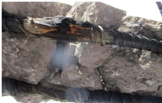
Figure 1. Uncovered HFRP Bars (by removing the clear cover after testing).
