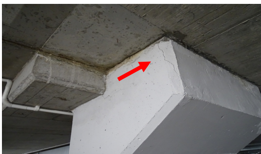
Fig. 2. Crack on the corbel edge.
