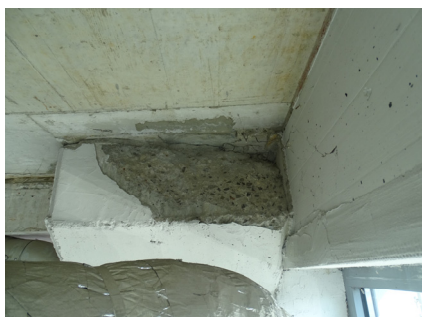
Fig. 1. Damage of the corbel surface.
