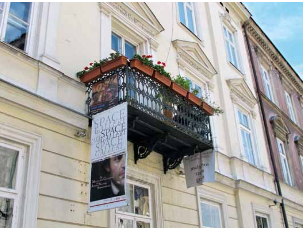
BANNER ATTACHED TO BALUSTRADE OF SIGNIFICANT HISTORICAL VALUE
