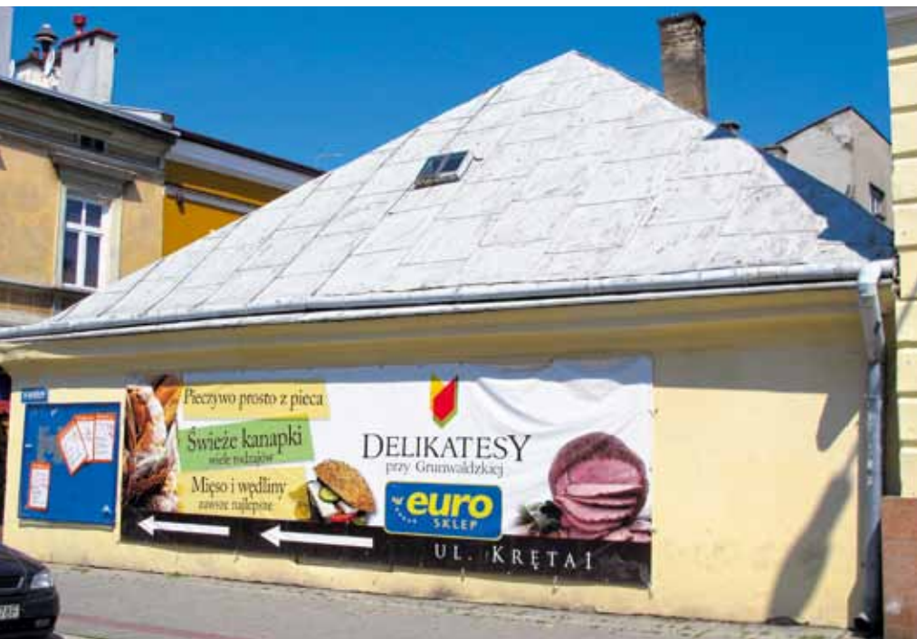
ADVERTISING BANNER COVERING TOO LARGE A PART OF THE ELEVATION
